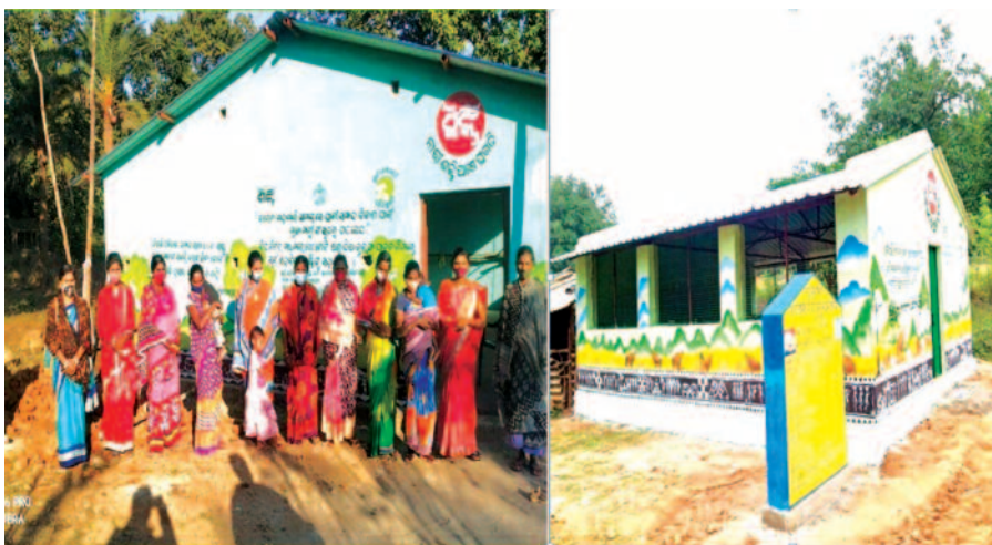
Construction of poultry shed of Maa Santoshi SHG at Talapada, Phiringia Block, Kandhamal District
